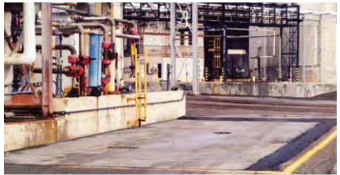
Secondary containment — Truck unloading pad with 3/8" non-skid topping
