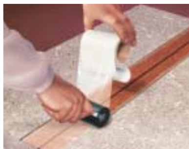
Crack /Joint Sealant System
